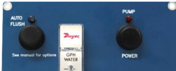
Figure 26: Operator Control Panel Detail
