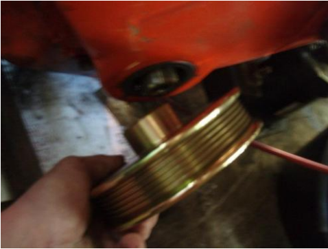
4. Grease the shaft, inside of the pulley and the lip seal. Install the new crank pulley
